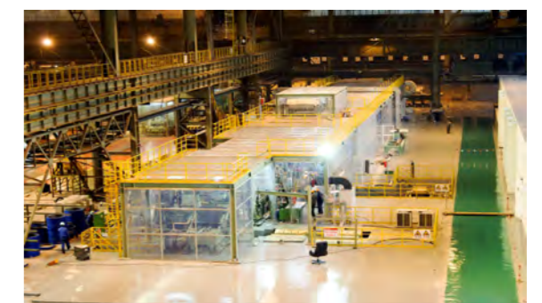
宝钢家电板重卷机组 BAOSTEEL appliance sheet recoiling line
